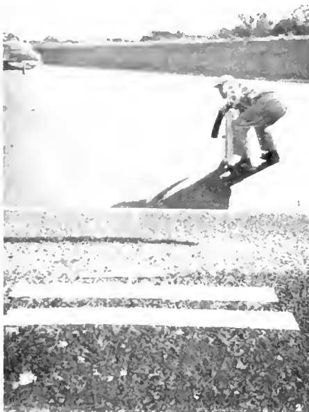
Placing strips on new plant-mixed surfacing to delineate traffic lane. Closeup showing pavement lane delineation strips adhering to rough-textured pavement. Pavement lane delineation strips placed immediately behind paving operations. General view of traffic lane markings.
